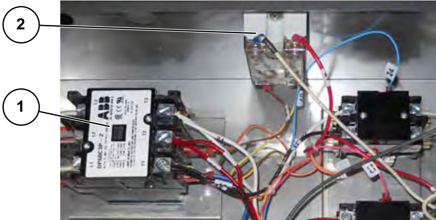
Electrical Components, Open Top View, Rear
